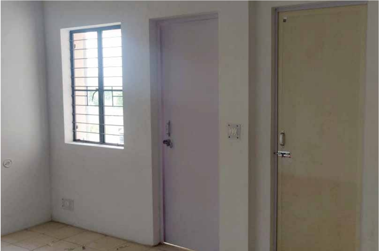
DLF GARDEN CITY, LUCKNOW EWS DOOR AND WINDOW
